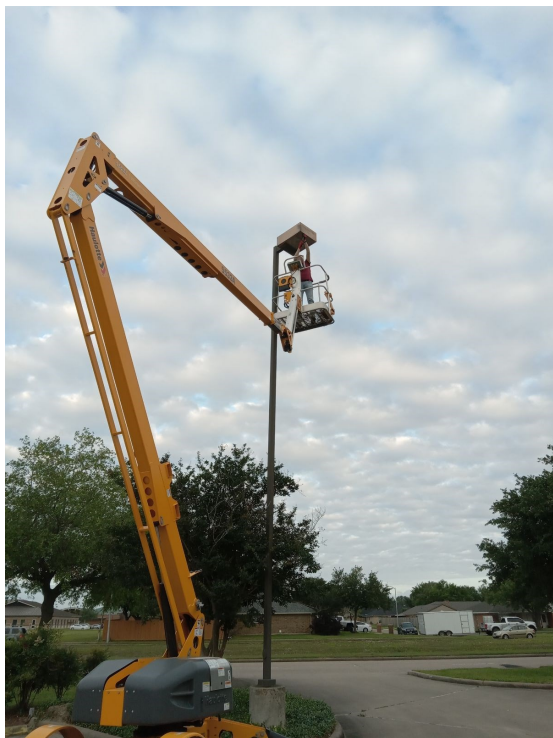
Brett Coe high up in the lift, changing light bulbs and keeping the parking lot safe and well lit. Thanks Brett!!
